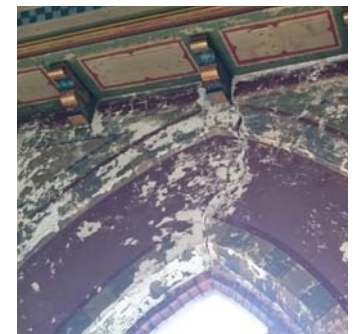
Figure 173. Crack in load-bearing wall
