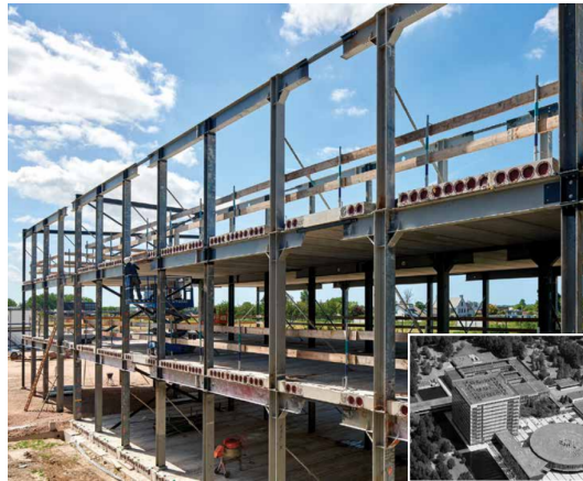
Figure 1.2: Construction of Biopartner 5, whereby steel elements are used from the neighbouring Gorlaeus-building (see below right) (Terwel et al., 2021)
