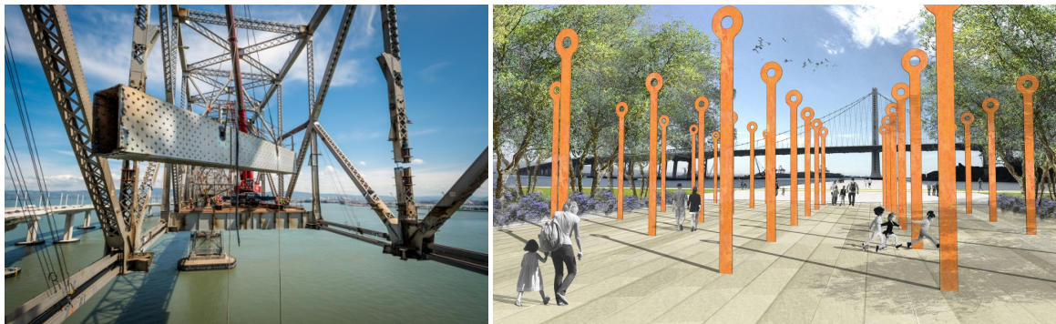
Figure 1.3: Left: Dismantling of the Bay Bridge (Oakland Museum of California, 2016) Right: The Field, an installation by CMG Landscape Architecture whereby steel bars from the Bay Bridge have been reused (Wakefield, 2017)
