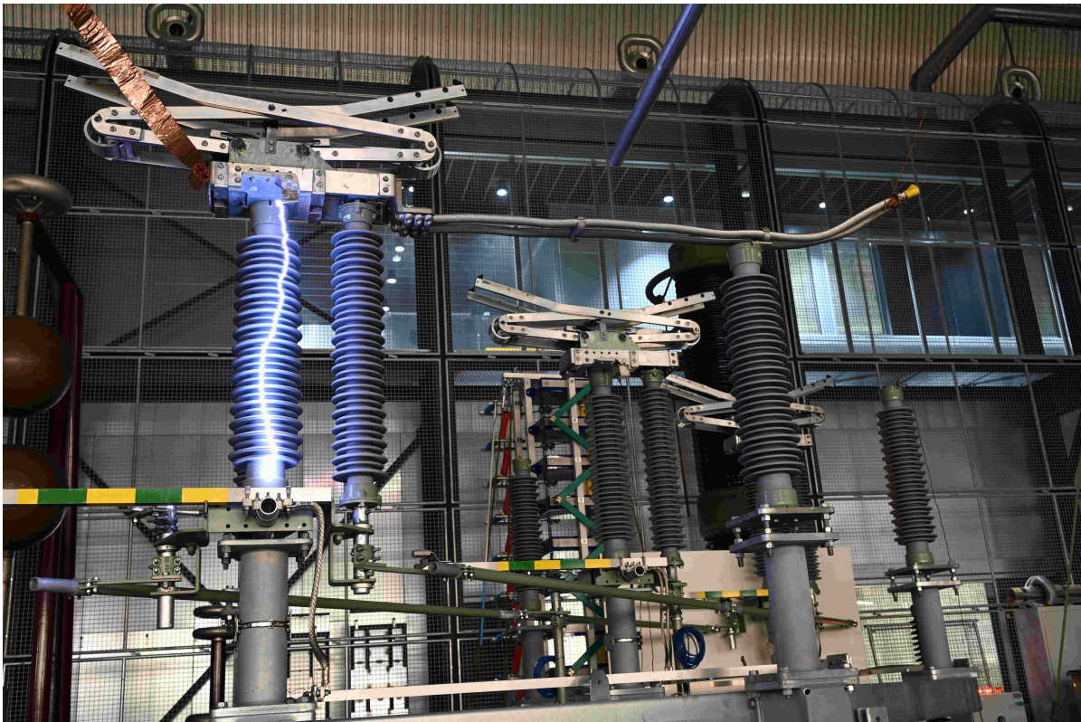
Figure 5.6: Flashover over the insulator
