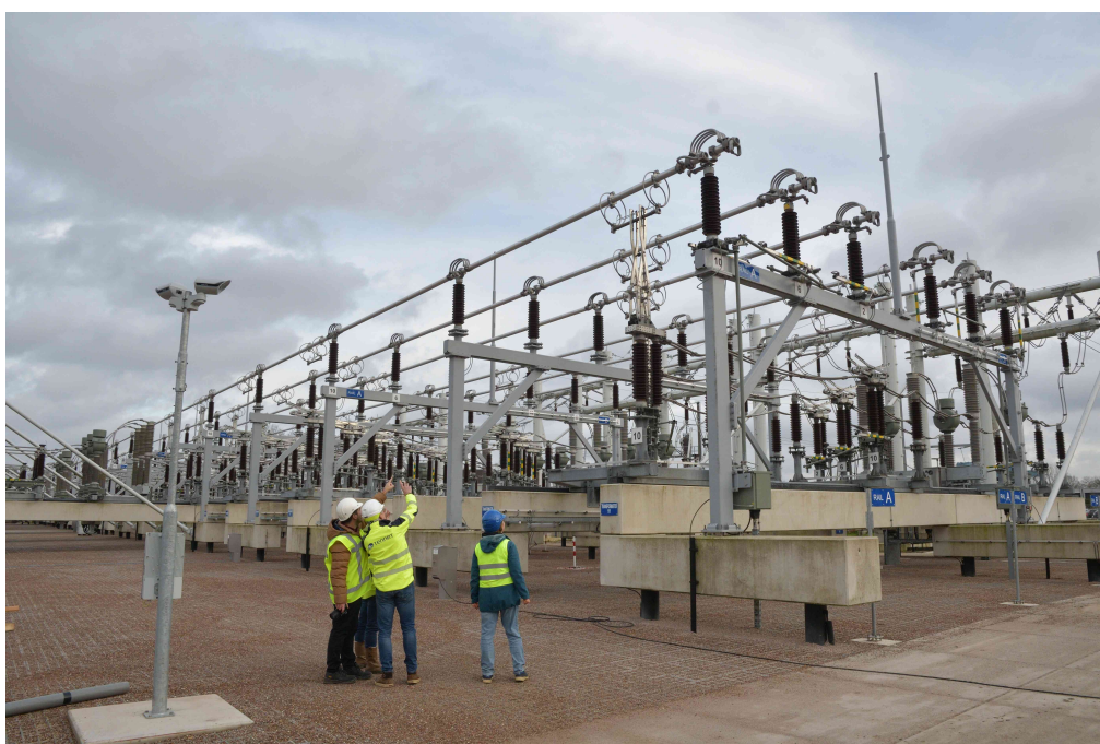
Figure 1.1: BRP substation with compact and modular bays. Image courtesy of C. Engelbrecht
