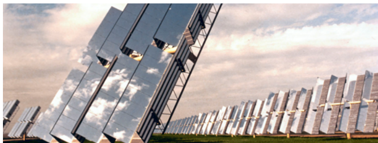
Figure 2.1: The world's first ever large-scale photovoltaic power plant in Carrisa Plains, California [16].
