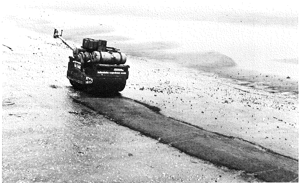
Photo 32 Repairing the seriously damaged surface of an asphaltic concrete revetment: The refilled area is compacted with a tandem vibratory roller
