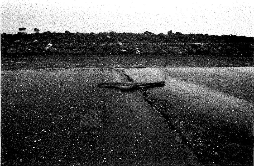
Photo 29 Because of a poorly constructed daily joint the subsoil material has been washed out causing the revetment material to deform
