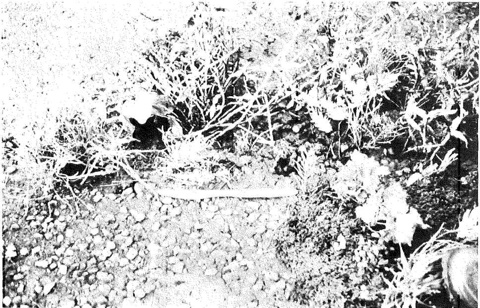
Photo 2 Plant growth damaging an asphaltic concrete revetment
