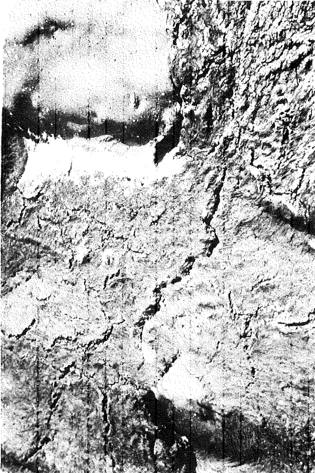
Photo 1 An asphaltic concrete revetment being attacked by algae
