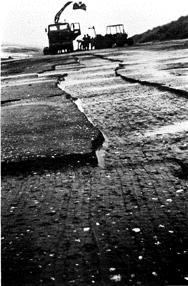
Photo 30 Repairing the seriously damaged surface of an asphaltic concrete revetment: The damaged area has been fraised out
