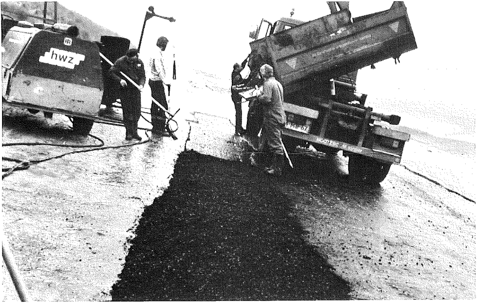
Photo 31 Repairing the seriously damaged surface of an asphaltic concrete revetment: The fraised area is refilled with asphaltic concrete
