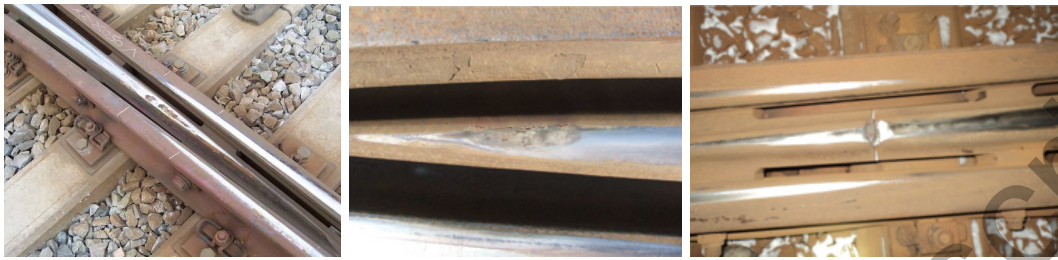
Figure 3 RCF damage to crossing nose
