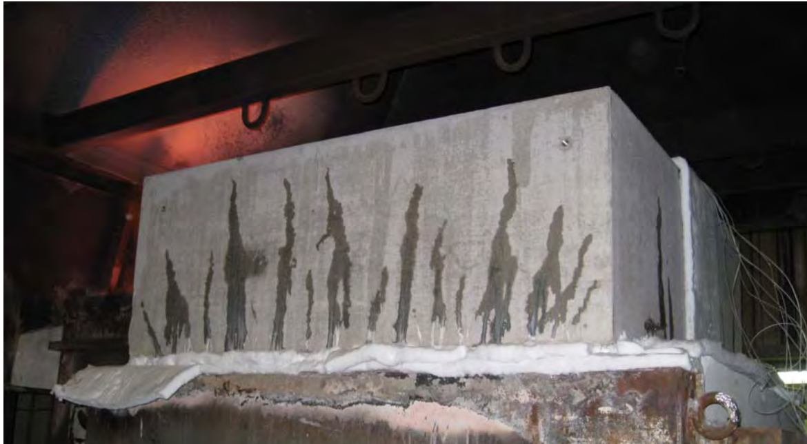
figure 15: leakage at outside of segment
