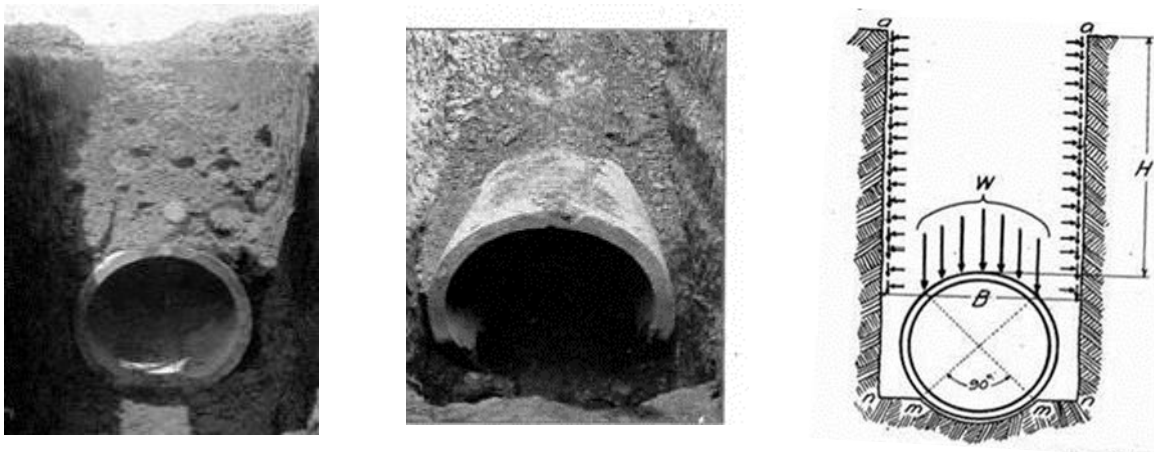
Figure A.2 BS8006 bases its calculation of load part A on the experimental research of Marston and Anderson (1913).
