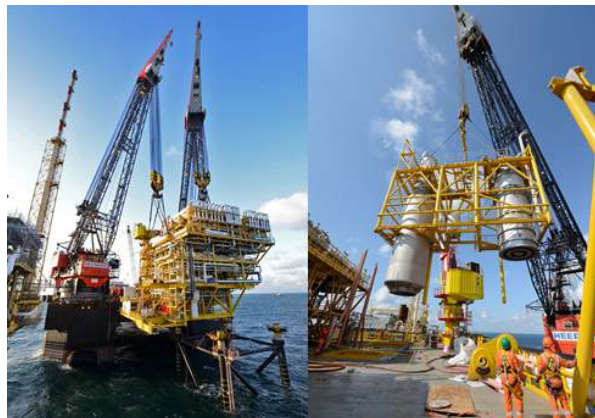
Figure 3.7: Heerema Marine Contractor its HLV Thialf installing a topside and system parts on the substructure
