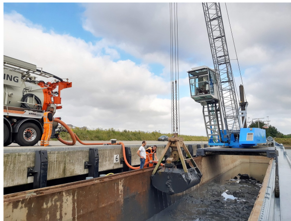
(c) Pumping the mud from the hopper into the truck for transport to Deltares.
