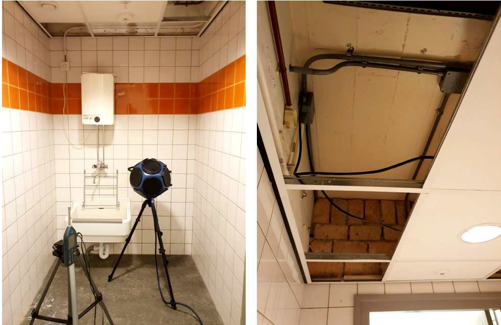
Figure 70. The room that is used to perform the measurement (left) and the removed panels of the suspended ceiling (right).
