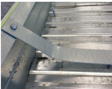
a) Strips c.t.c. 500 mm to prevent bending of the joist shuttering due to wet concrete.
