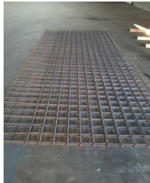
b) Reinforcement meshes, sufficient in size to cover the entire test specimen and to avoid overlap
