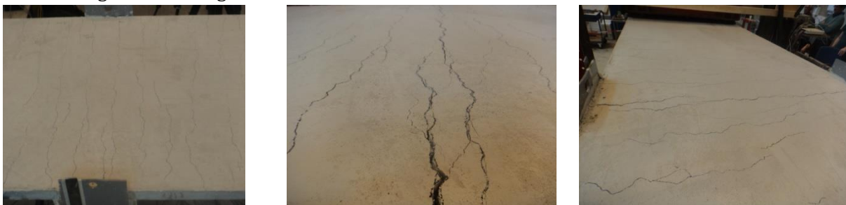
Figure H 3 Crack pattern specimen 1, final failure at the middle of the steel beam
