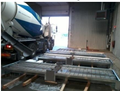
a) Pouring of the concrete, all specimens will be casted at once.
