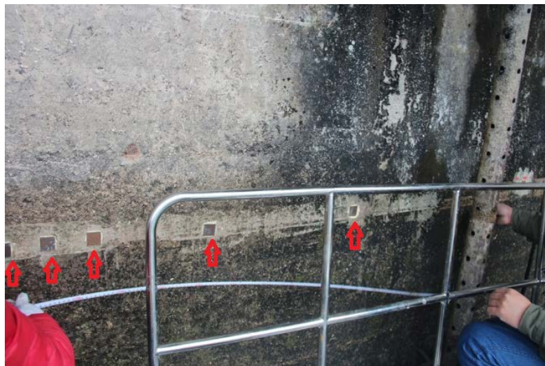
Figure 2: Sensor location on the dam surface (pointed by red arrow)
