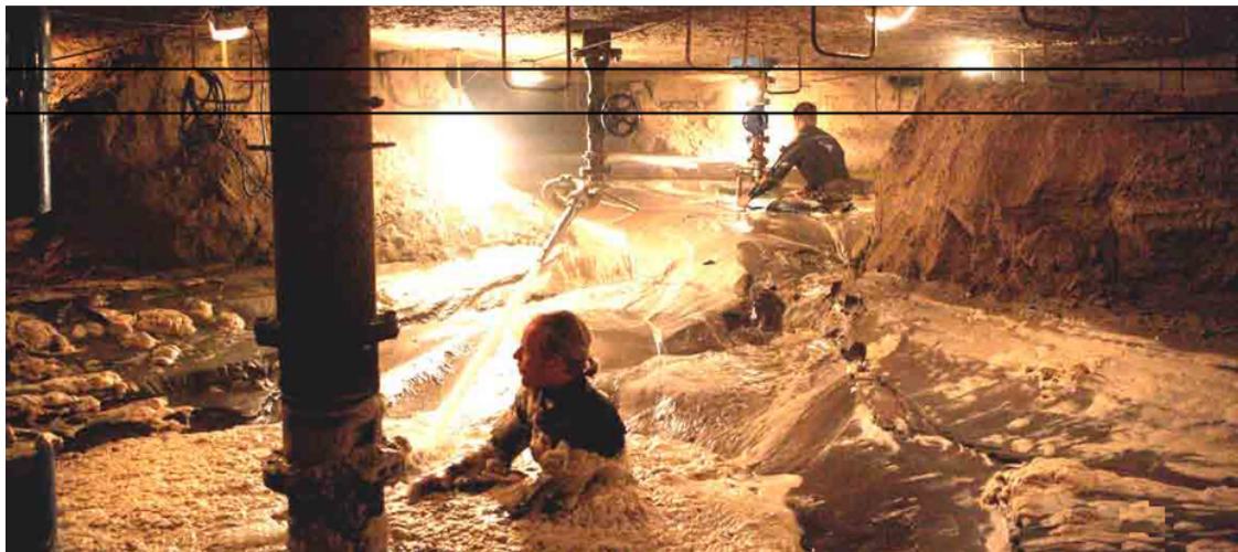
Figure 5.8: Photo of the inside of the working chamber of a pneumatic caisson [Pepers, 2011]
