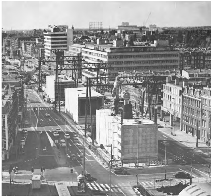
Figure D.7: An old photo from the pneumatic caissons on surface level used for the Oostlijn [Ouwendijk, 1977]
