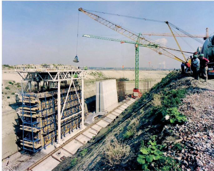
Figure 7.13: Quay wall constructed under dry conditions in a building pit with a dewatering system [De Gijt et al 2003]
