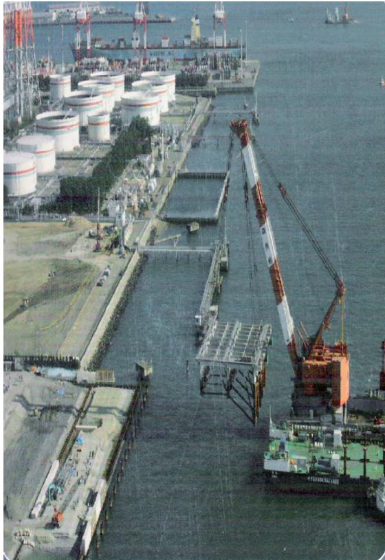
Figure 7.26 Heavy lifting crane used for placing the steel top on the installed piles [Hoshiyama 2009]
