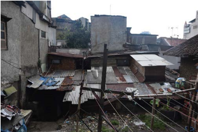
Lack of means to repair homes
