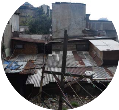
Poor housing construction
