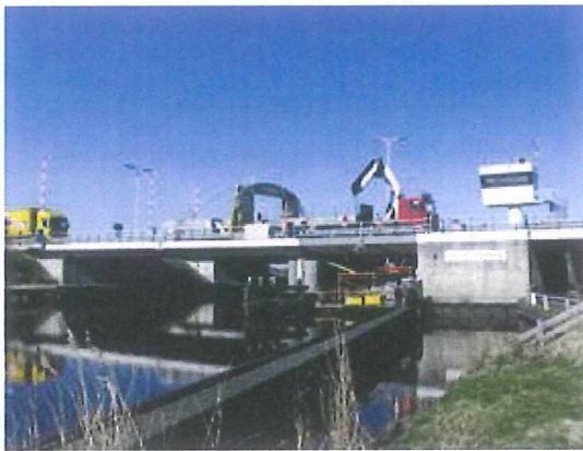
Figure 1 – Scharsterrijn Bridge (fixed part on the left side and movable part on the right side).
