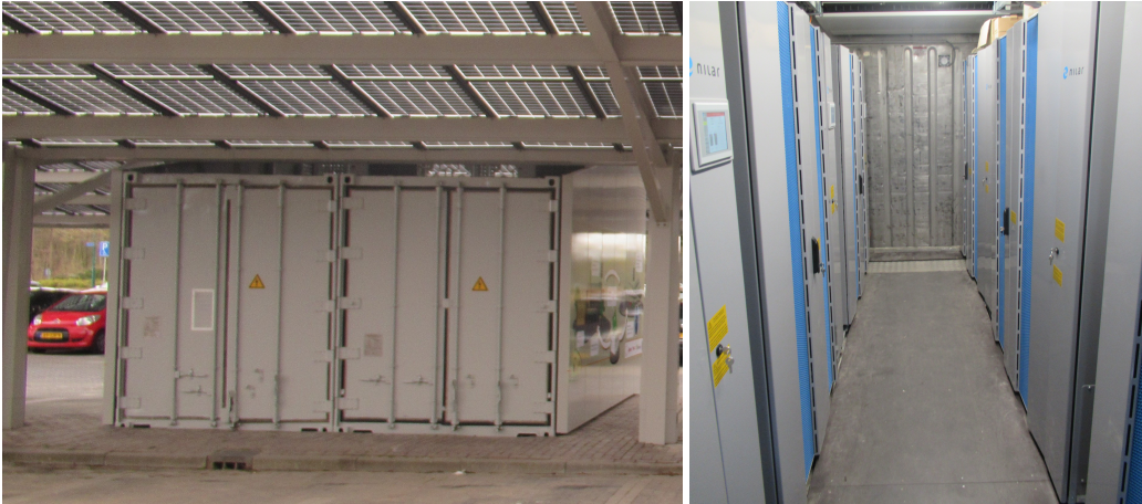
(a) Battery housing located under the carport roofs (b) Battery cabinets within the housing
