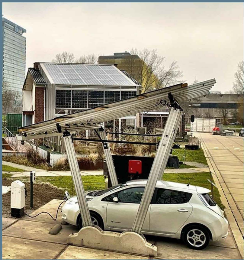
A solar carport with vehicle-to-grid (V2G) charging at the Green Village, TU Delft
