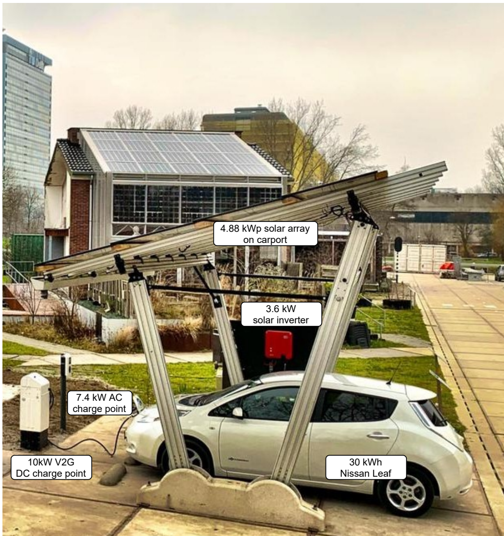
Figure 7.3: V2G test set-up at the solar carport located at the Green Village, TU Delft (Image courtesy of The Green Village)
