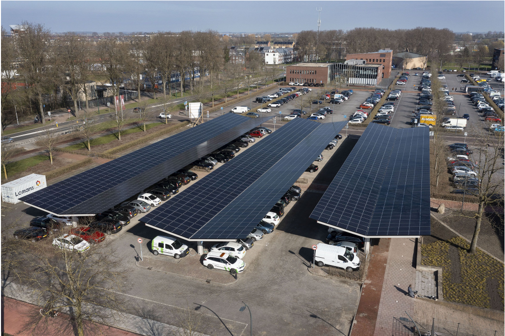
Figure 1.4: Solar carports for EV charging constructed at the municipality building, Dronten, the Netherlands
