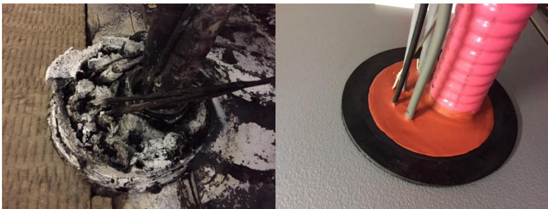
Figure 45 – Two sides of NOFIRNO® transit after a fire
