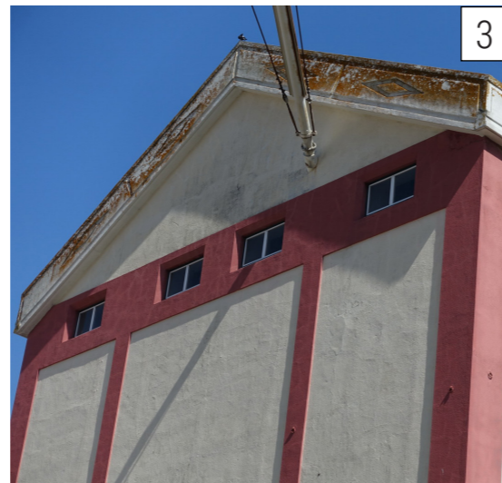
Building 18: the eaves are in a bad condition due to water damage (relief).
