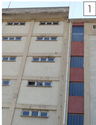
Building 20: part of the water pipe is missing causing leakage.
