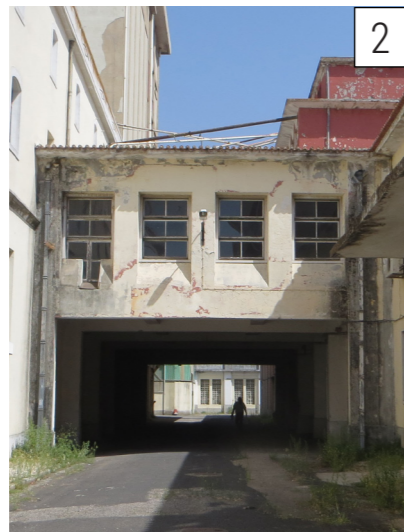
Building 16B: this building part causes water damage around the drainage system.
