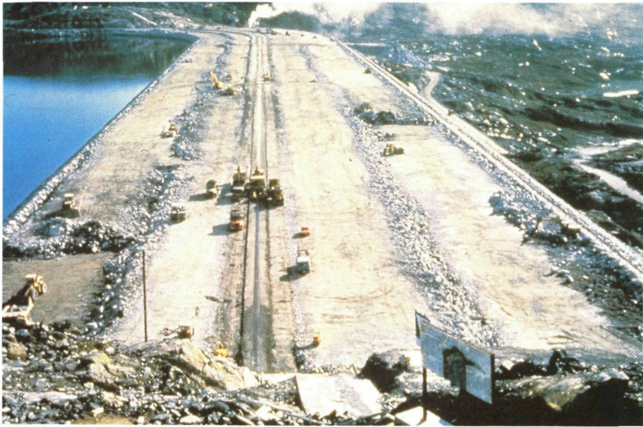
Fig. 6.1 The thin asphaltic concrete core adjusts to the deformations in the embankment (from the construction of Storvatn Dam)
