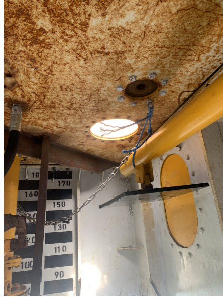
Figure 6.17: Floater attached to top of the CDS
