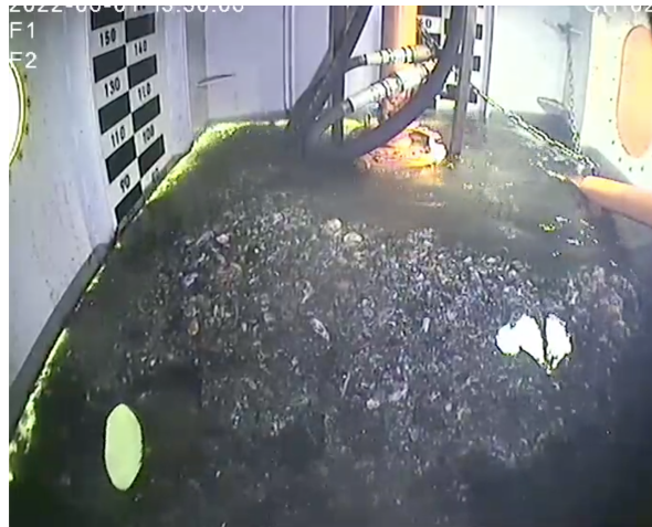
Figure 6.12: Photo inside chamber with pump on
