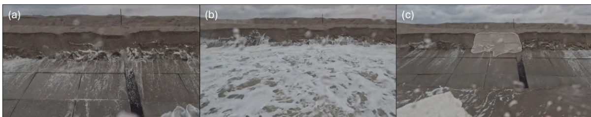
Figure 4.10: Slumping event observed by GoPro_01 during high water 2.b on 22 December 2024. Sequential frames show the collapse of the dune face and sand movement over a two-second interval: (a) 08:38:29, (b) 08:38:30, and (c) 08:38:31. This illustrates the dynamics of mass failure under wave loading.
