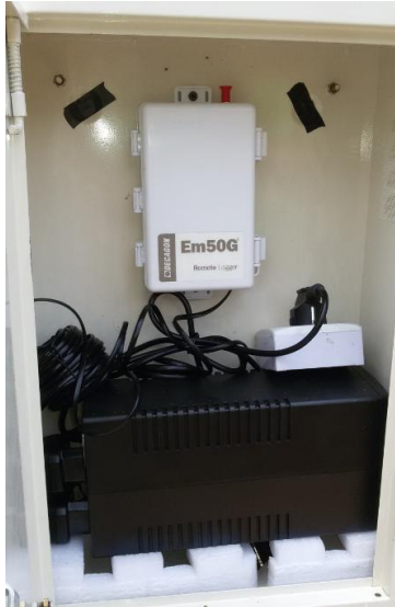
Figure 16: Overview of the electricity box, with an UPS system and the data logger of the tipping bucket
