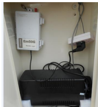
Figure 21: Overview of the electricity box, with an UPS system and the data logger of the tipping bucket
