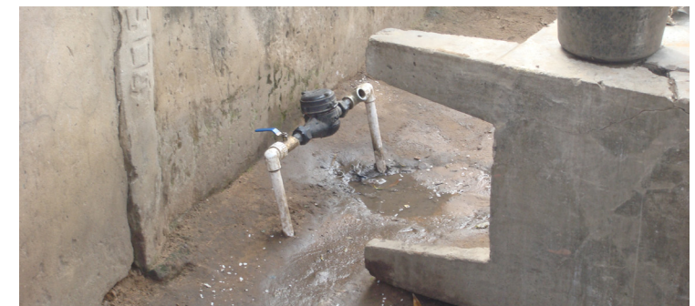
Figure 4.9: water supply with meter, shared by three families, Mafalala neighbourhood, Maputo. (EW)
