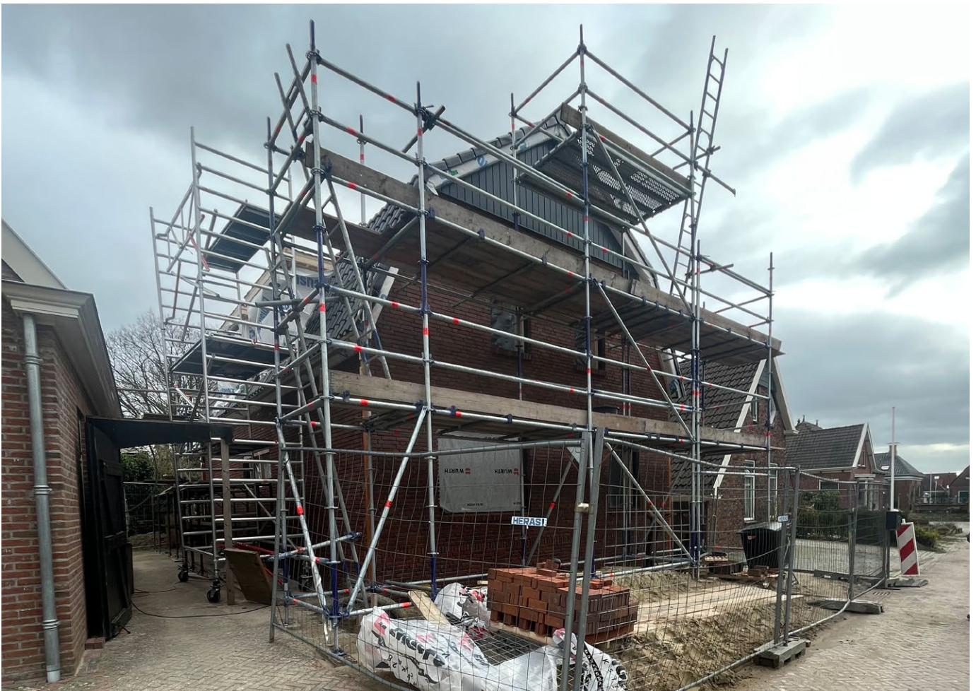
Figure 4: Example of building and street reinforcement project in Loppersum, Groningen. Sophia Arbara
