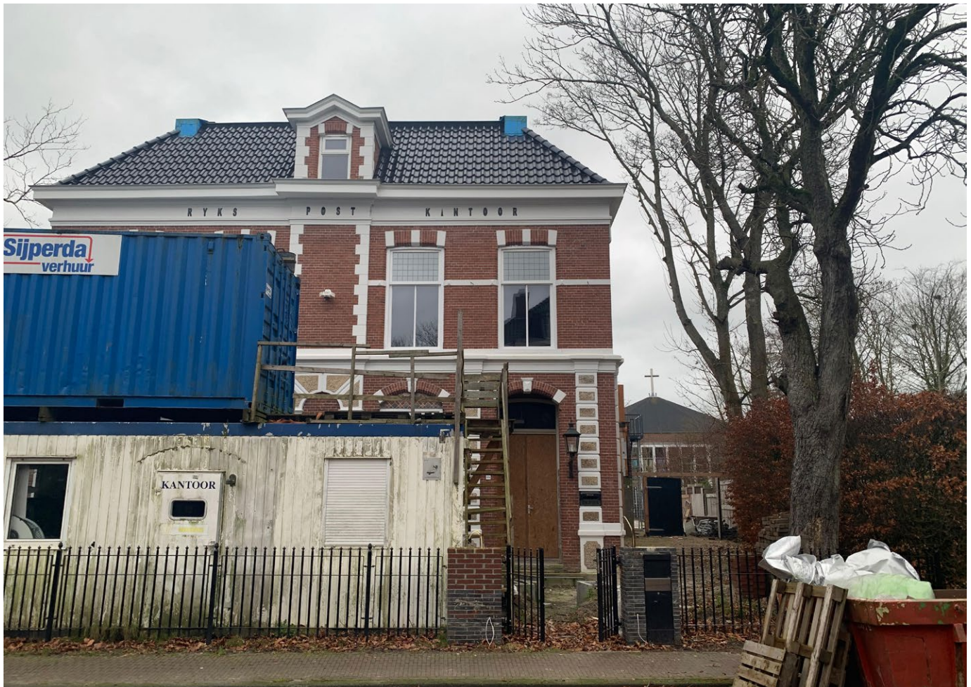
Figure 1: Long process of reinforcement of monumental building, Raadhuisstraat 5, Loppersum. NCG Atelier Regiobouwmeester
