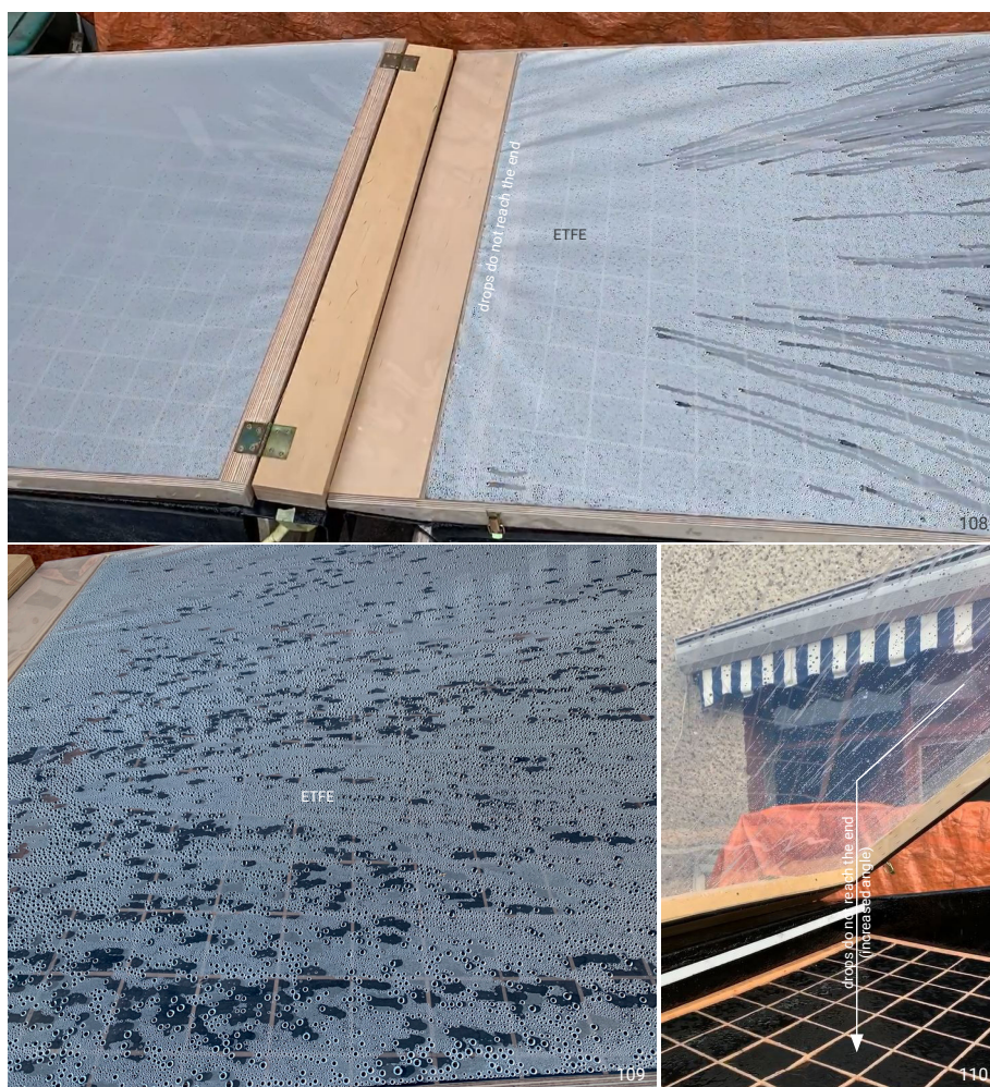
Phot. 108-110 ETFE fail test. Author's photography.
