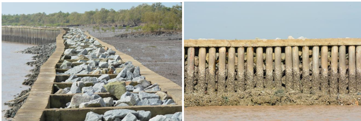
Figure L3: Concrete breakwater as build along the West Mekong Delta shoreline(J. Wölcke et al., 2016)
