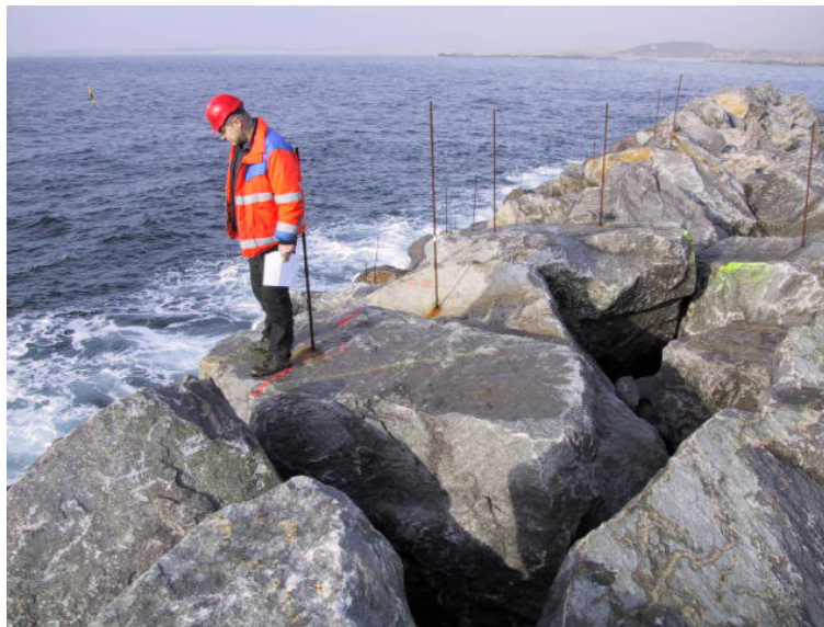
Figure 1.3 Inspection of the front slope of the berm of the Sirevåg breakwater, a section with Class I stones. Sigurdarson et al 2001
