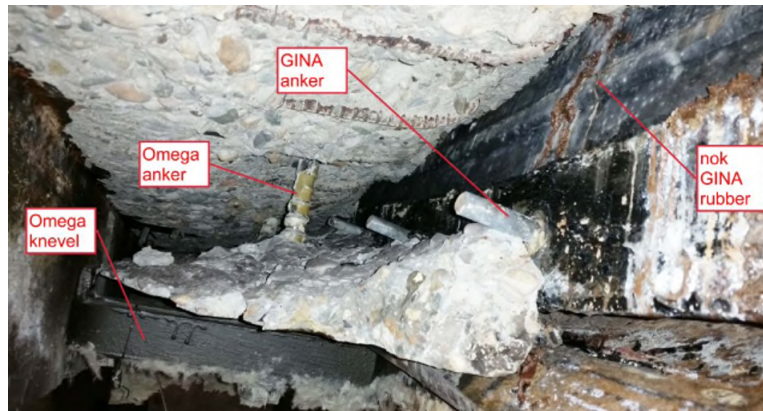
Figure 2-2: Damage picture in early 2015 showing damaged Gina gasket and Omega seal of Rotterdam Metro Tunnel (Molendijk et.al, 2019)
