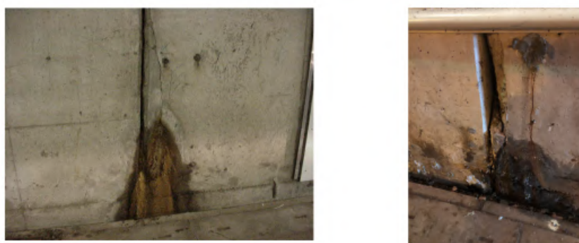
Figure 2-15: Leaky expansion joint with crack in concrete cover of Kil Tunnel identified in 2001 (left) and in December 2019 (right) (Yang, 2020)
