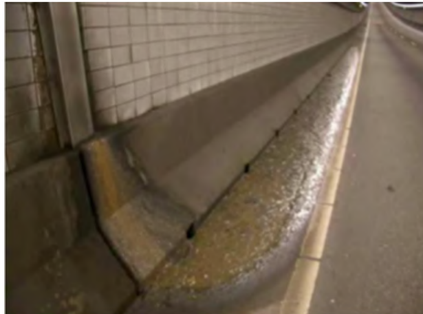
Figure 2-5: Sand and water leak in east tube of First Coen Tunnel (Leeuw, 2008)
