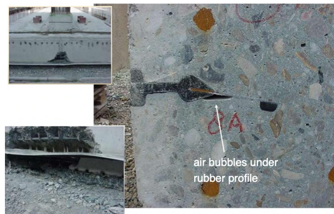
Figure 2-35: Lack of workmanship during concreting (Leeuw, 2013)
