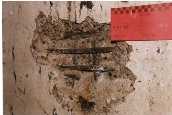
Figure 2-10: Reinforcement corrosion from inspection in 1988 (SEG, 2019)
