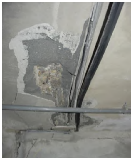
Figure 2-29: Delaminated concrete (Schols, 2012)
