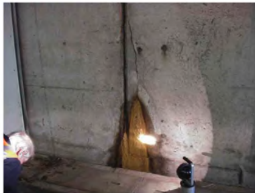
Figure 2-12: Cracking at expansion joint of Kil Tunnel (Gavin et al., 2019)
