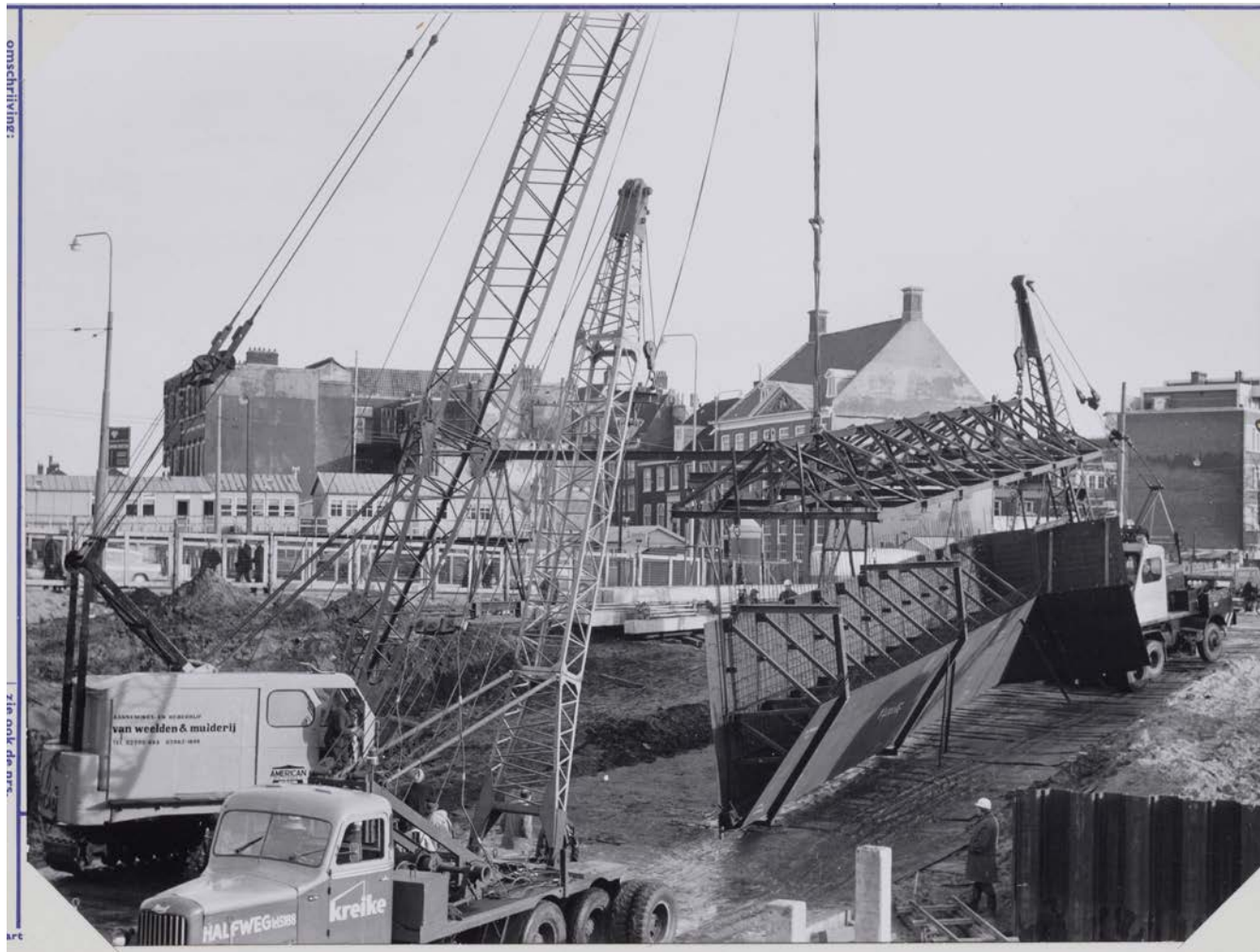
Part of the steel cutting edge for caisson is driven into the pit.
