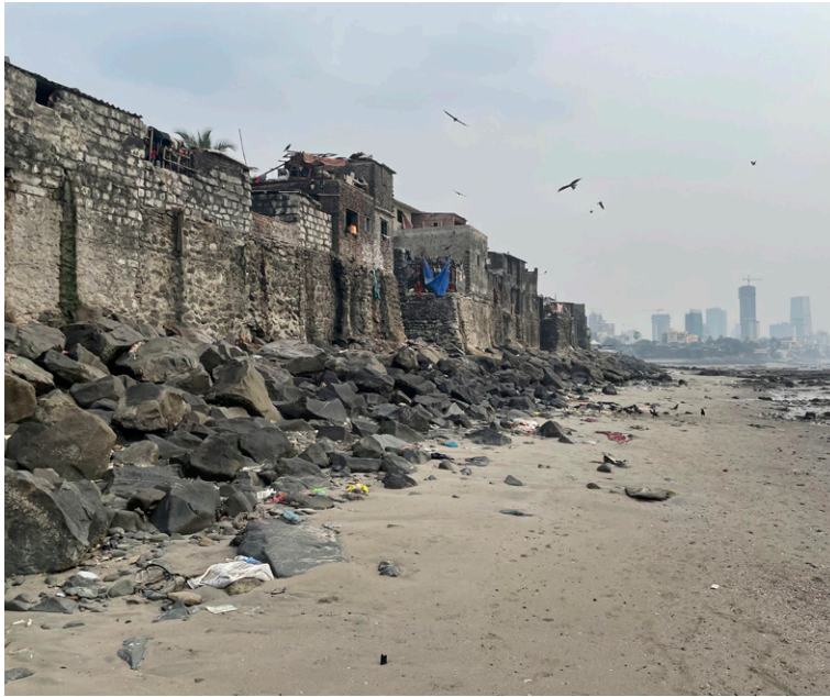
BLUE | Hydromorphology compromised - Sea Walls resulting in rise of ground water level with salt water intrusion
