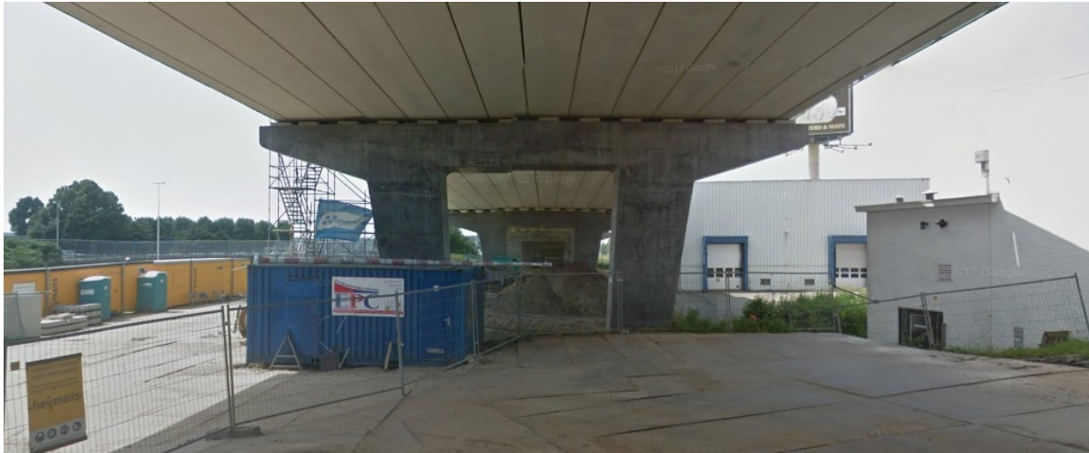
Figure 4-8 Bottom view of N451. Located on the south embankment of the Amalia bridge. Facing in the south direction. (Google Streetview, 2017)
