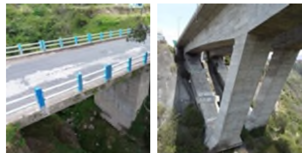
Figure 6. Sample images captured using the UAV on case study bridge 1 (left) and 2 (right)
