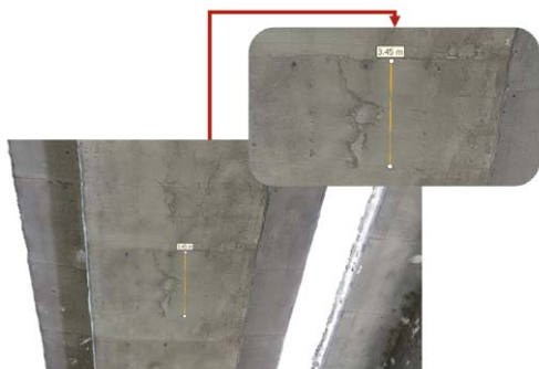
Figure 9. Damage measurements of Case Study 2
