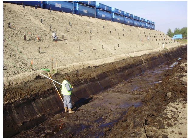
Fig. 5. Investment in innovative monitoring and performance understanding for a dyke reinforcement programme. Courtesy: Rijkswaterstaat.
