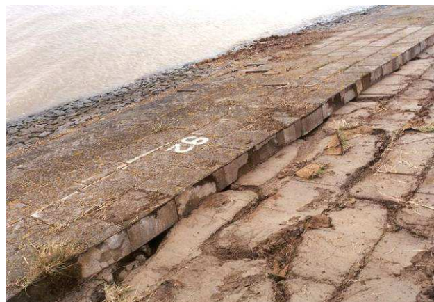
Fig. 7 Gullies under the blocks in the clay subsoil
