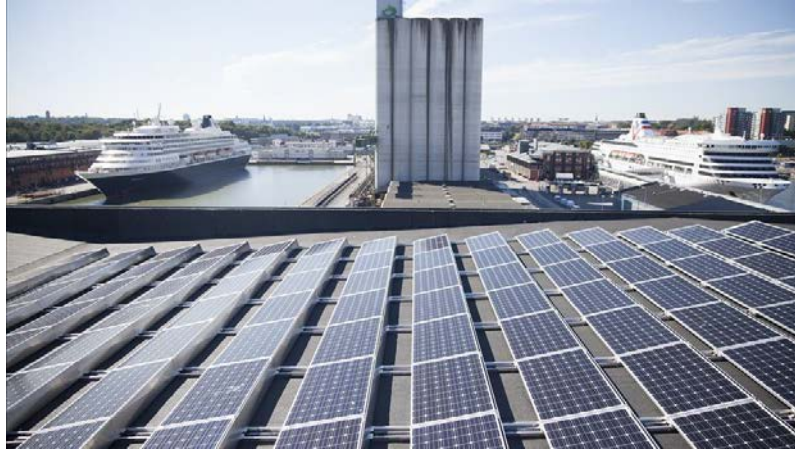
Figure 18 Photovoltaic Installation in Stockholm Port (Stockholms stad, 2014)
