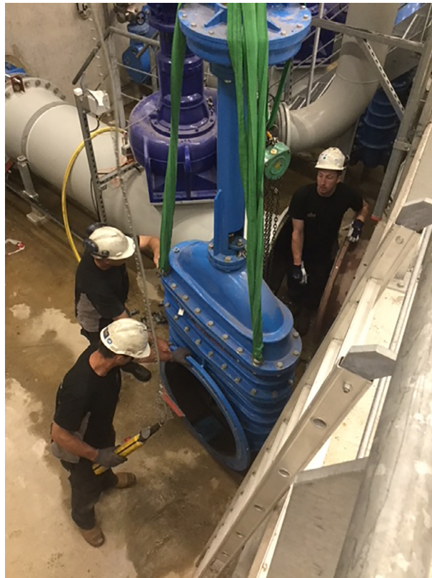
Fig. 4 Expanding the valve casing at Ramspol Barrier. (Image: Courtesy of Rijkswaterstaat, Tycho Busnach.)
