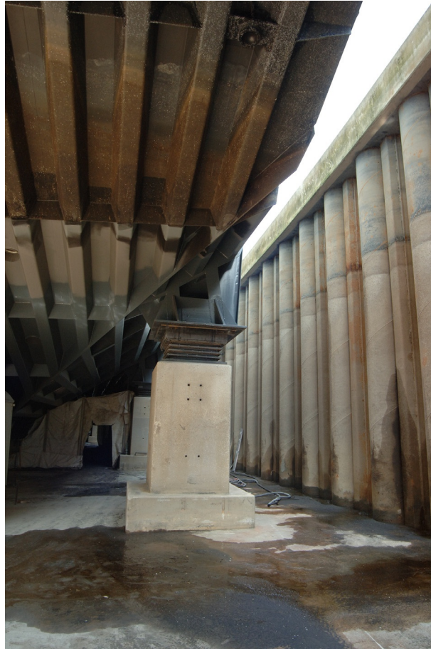
Fig. 2 Compression blocks under the gate at Maeslant Barrier. (Image: Courtesy of Rijkswaterstaat.)
