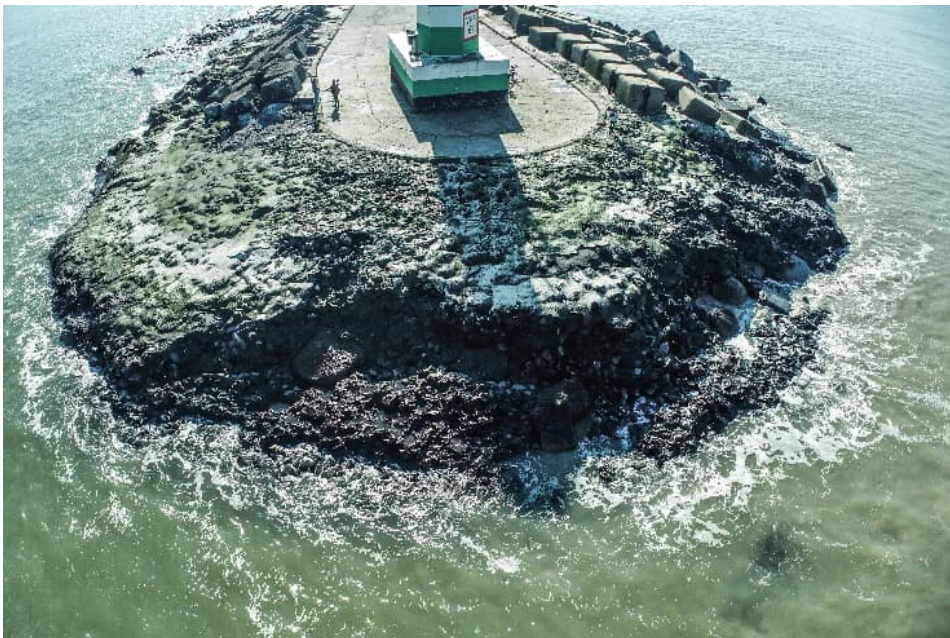
Figure 1.3: The Southern Breakwater at IJmuiden showing the configuration of asphalt and armour blocks. This image was taken in 2023 following storm damage. Repairs have since been executed (Rijkswaterstaat, 2023).
