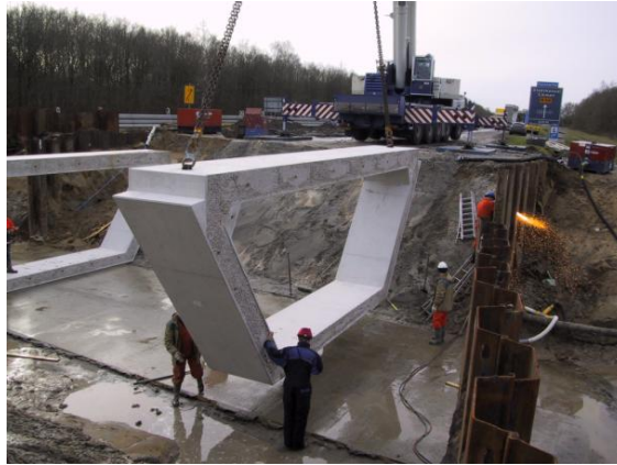
Figure 10.1: Lifting the prefab concrete element into its final position, photo by Romein Beton BV
