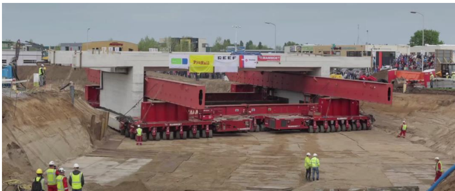
Figure 10.2: Driving the completed structure into its final position, picture taken from time-lapse movie of Didam - Youtube © [58]
