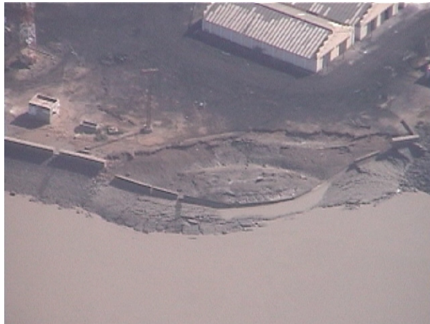
Figure B.11 Earthquake-related failure of the coastal protection at Navlakhi port, India 2001 33
