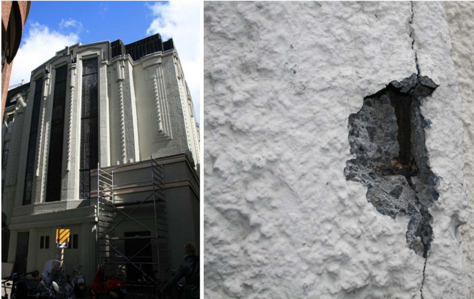
Fig. 4. One of the first Dutch buildings with exposed concrete, yet currently painted (architect A. Moen, 1915). Left: Overview of the rear façade. Right: Detail of a pilaster with spalling, cracking and corrosion, showing the original concrete made with crushed porphyry and with a tooled surface under a layer of paint.
