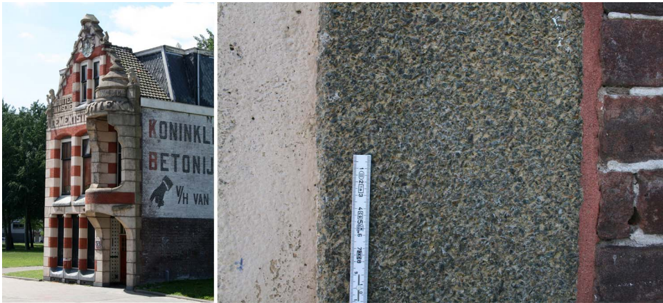
Fig. 2. Former head office of the artificial stone company Rotterdamsche Cementsteenfabriek Van Waning & Co (1898). Left: Overview of the main façade with artificial stone elements painted white. Right: Detail of the corner showing the original, tooled concrete surface made with greenish aggregate.
