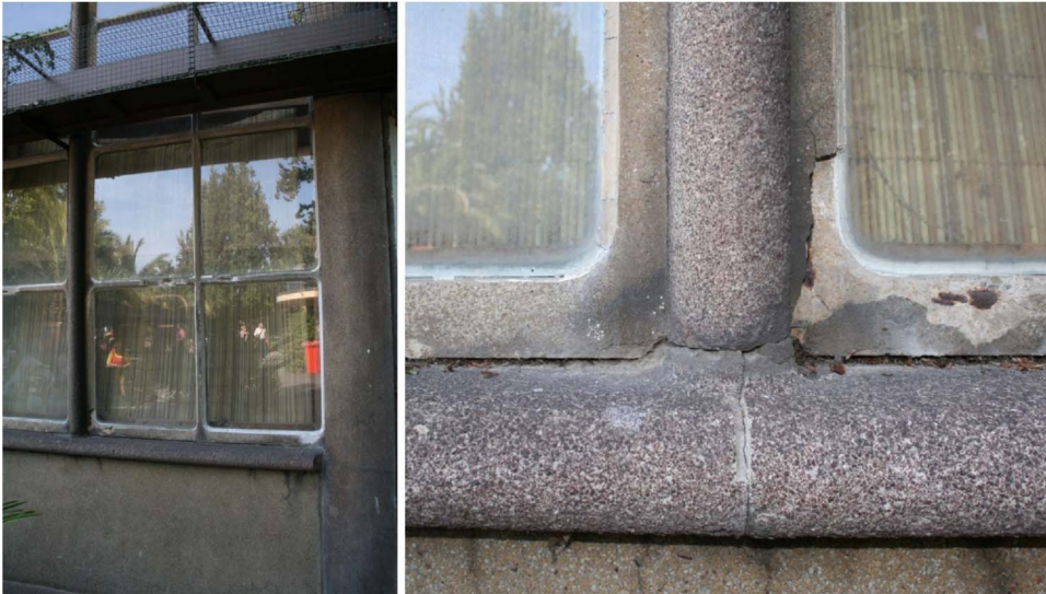
Fig. 5. Precast concrete elements (window frame and sill, plinth, columns etc.) made by Schokbeton N.V., using different ground aggregates to alter the colour of the concrete (Zoo Blijdorp, architect S. van Ravesteyn, 1939). Left: overview façade. Right: beige-sandstone coloured window frame and a more pink-purple coloured windowsill and column. Partially spalling and cracking has occurred, exposing the reinforcement, and discolouration due to soiling.
