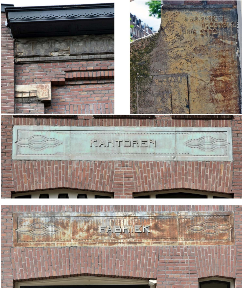
Fig. 3. Overview of precast metallised concrete elements in a former factory (architect C. Tenenti, Amsterdam, 1921). Top left: Cornice made with dark coloured concrete and capital with a sand stone coloured metallised concrete with local darker patches. Top right: detail of a yellow-brown coloured base, with visible inscription of the year and patent number. Middle: Green copper coloured precast metallised concrete sign above entrance for offices. Bottom: Multicolour (green, rust coloured) sign above the entrance to the factory.
