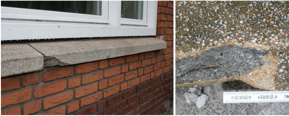
Fig. 6. Typical mass-produced precast concrete windowsill dating from the 1930s. Left: Overview of a windowsill with a broken off corner. Right: Close-up of a damaged windowsill showing a coloured facing layer and a grey backing concrete. Due to soiling, the original colour changed from a beige-orange colour to a more dirty shade of green.
