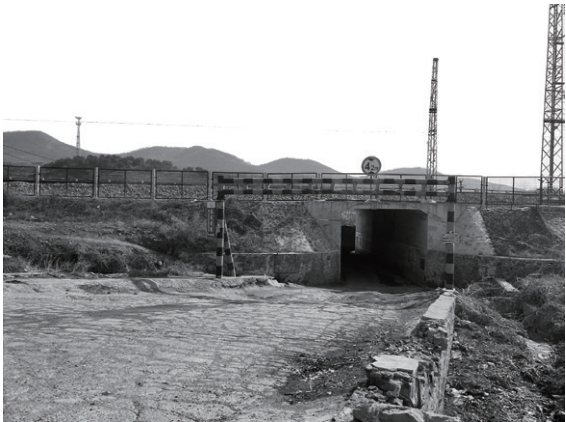
Low Quality of underpass Photographed by author
