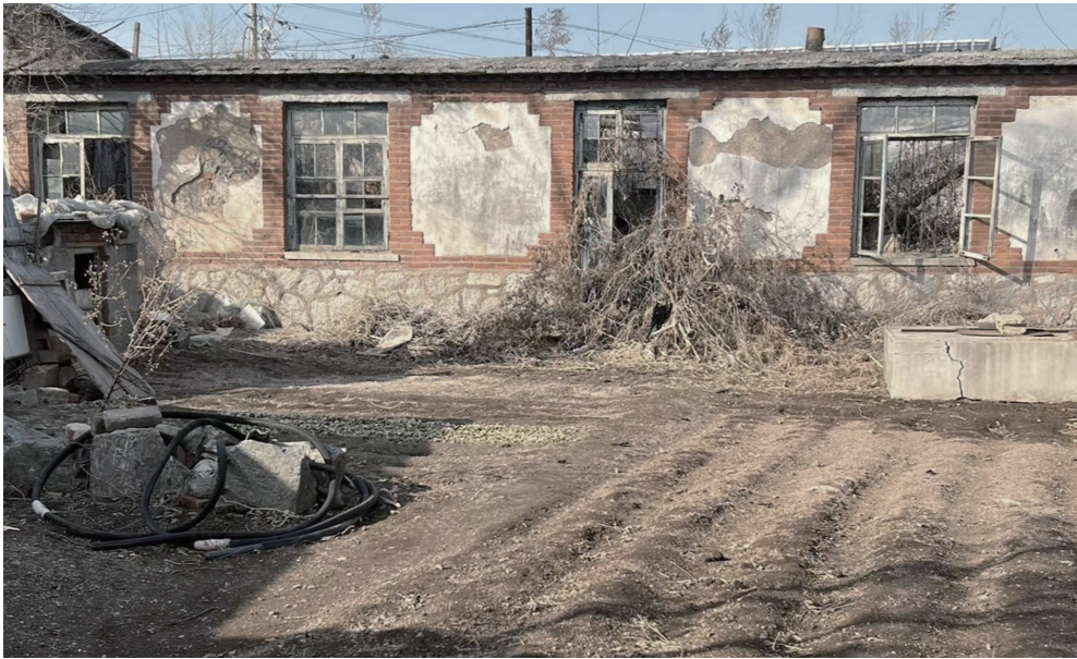
Abandoned houses in low condition Photographed by author
