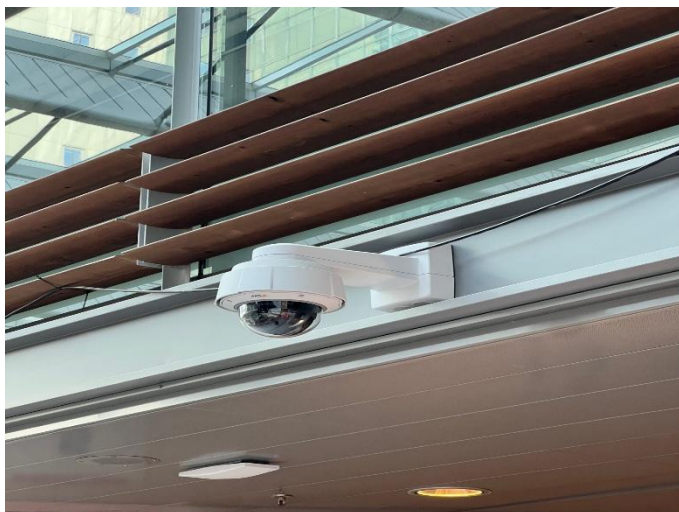
CCTV camera in atrium roof structure
