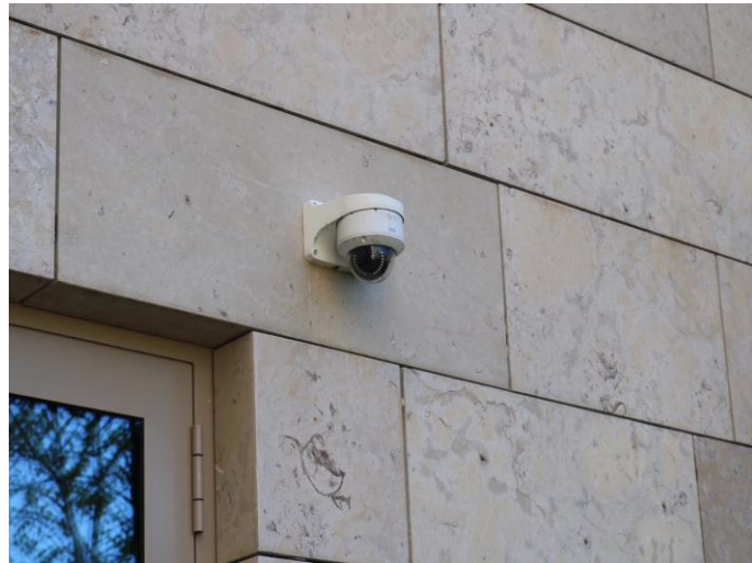
CCTV camera on facade
