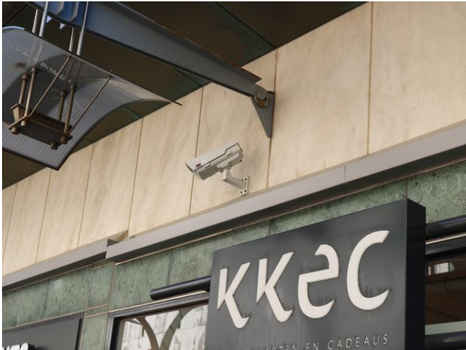
CCTV camera above retail unit
