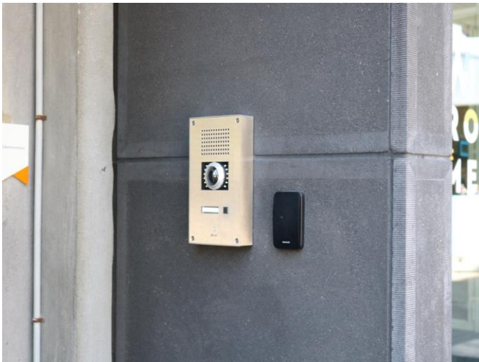
Intercom and key card reader at secondary entrance
