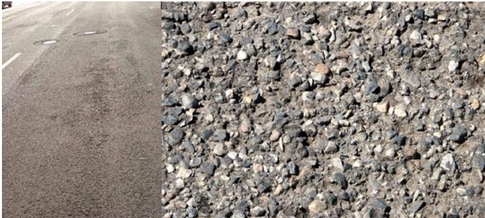
Figure 22, loss of material due to ravelling (Ahmad & Khawaja, 2018)
