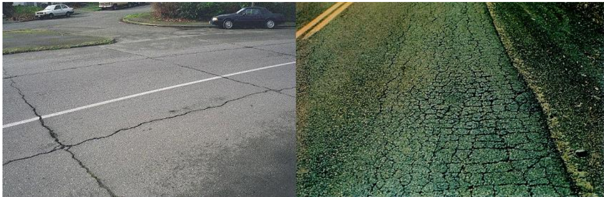
Figure 28, left reflective cracking and right alligator cracking (Pavement Interactive, 2020).
