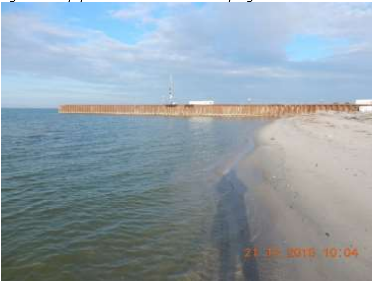
Figure 0-6 The water line and in the background the sheet-pile wall is observed
