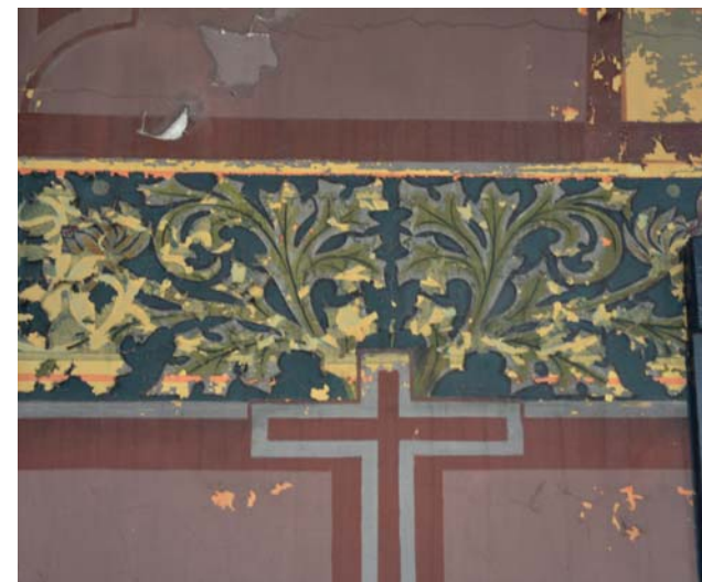
Figure 21. The strip, paintwork peeling and revealing
