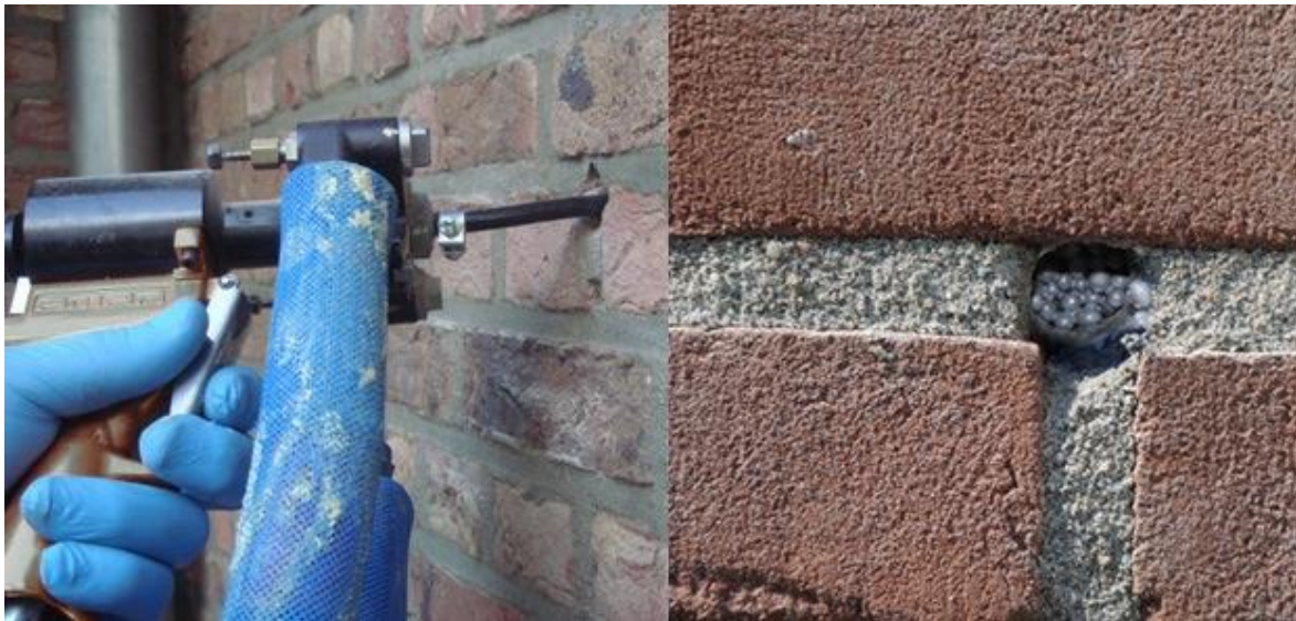
Figure 42: Hole in the mortar to fill the cavity with EPS pearls. Reprinted from (Isolatie-info.nl, n.d.)
