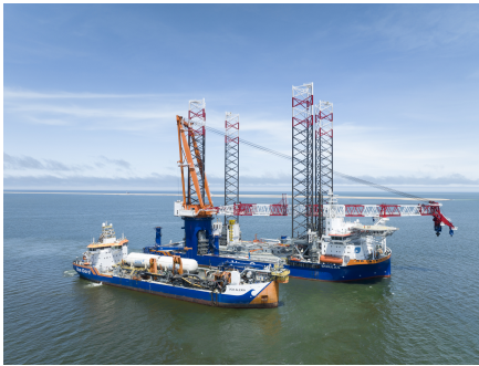
(a) Trailing suction hopper dredger Vox Alexia (front) and offshore installation vessel Boreas (back) [313]
