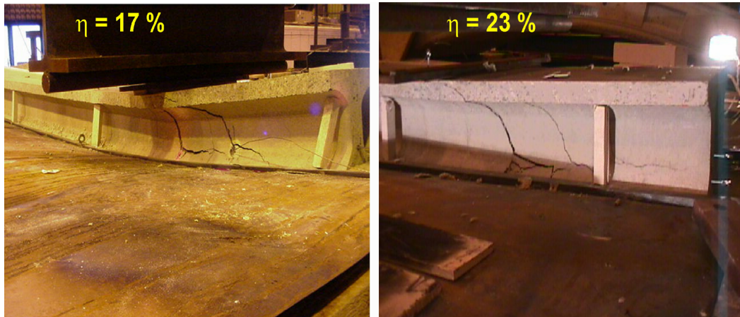
Figure 4.12: Crack pattern after failure in two HVP260 tests, seen from the side with a strand in the rib at 76 mm from the exposed side.
